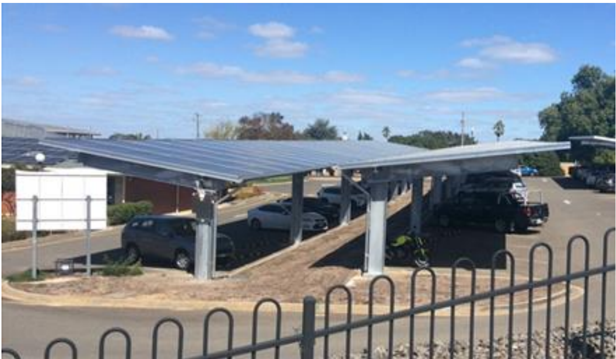
Figure 1. Carpark shading with integrated solar panels at Ararat Hospital
